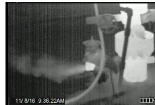
Leak from a wellhead only visible with an infrared camera
